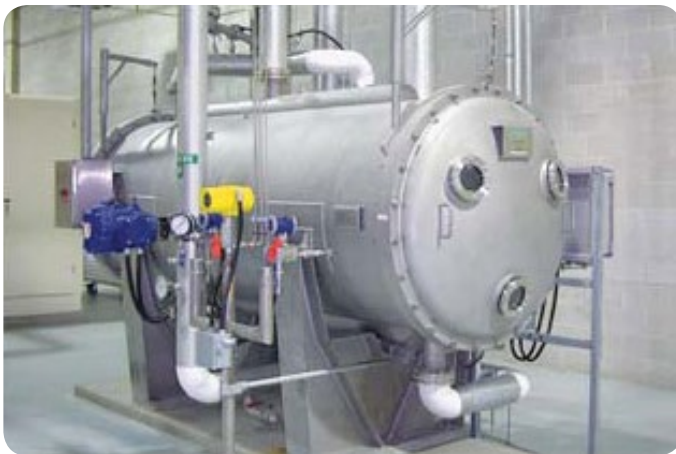
The Ozone generator 2
